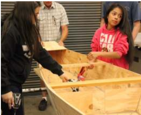
High School Industrial Arts: carpentry, metal shop, and welding classes restarted recently thanks to our donors!
